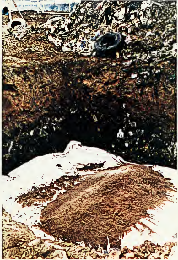
A3: GARBAGE REMOVED TO REQUIRED DEPTH. FILTER CLOTH INSTALLED. FIRST LAYER OF SAND APPLIED.
